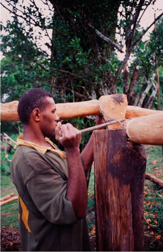
Architecture of Fiji, Fig. 39 Man in Navala village fixing a wall plate to a pile with wire. In former times such a joint would have been lashed with lianas or coconut cord
