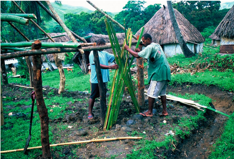
Architecture of Fiji, Fig. 36 Woven bamboo walls are attached to the sides of the building
