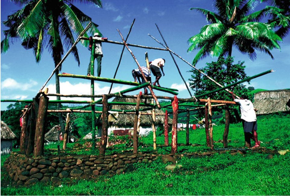
Architecture of Fiji, Fig. 35 After placing the wall plates, a temporary bamboo scaffolding is set up in the middle of the house. This holds the roof ridge, until the rafters are fixed to it
