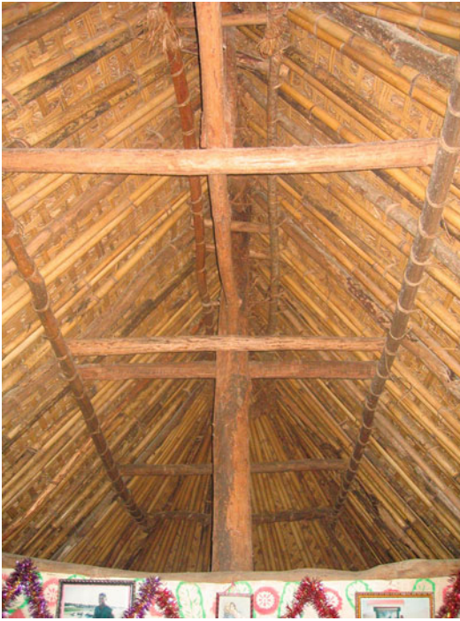
Architecture of Fiji, Fig. 45 Inner roof structure of a house in Navala village (Source: Josef Schuller)
