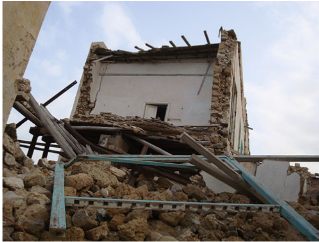
Architecture in Suakin, Fig. 4 View of the upper storey of a partly collapsed house on Suakin Island, exposing its construction techniques. Note the large dressed surface blocks of the wall and its rubble infill and thick multilayered upper floor. The light-green rectangular wooden
