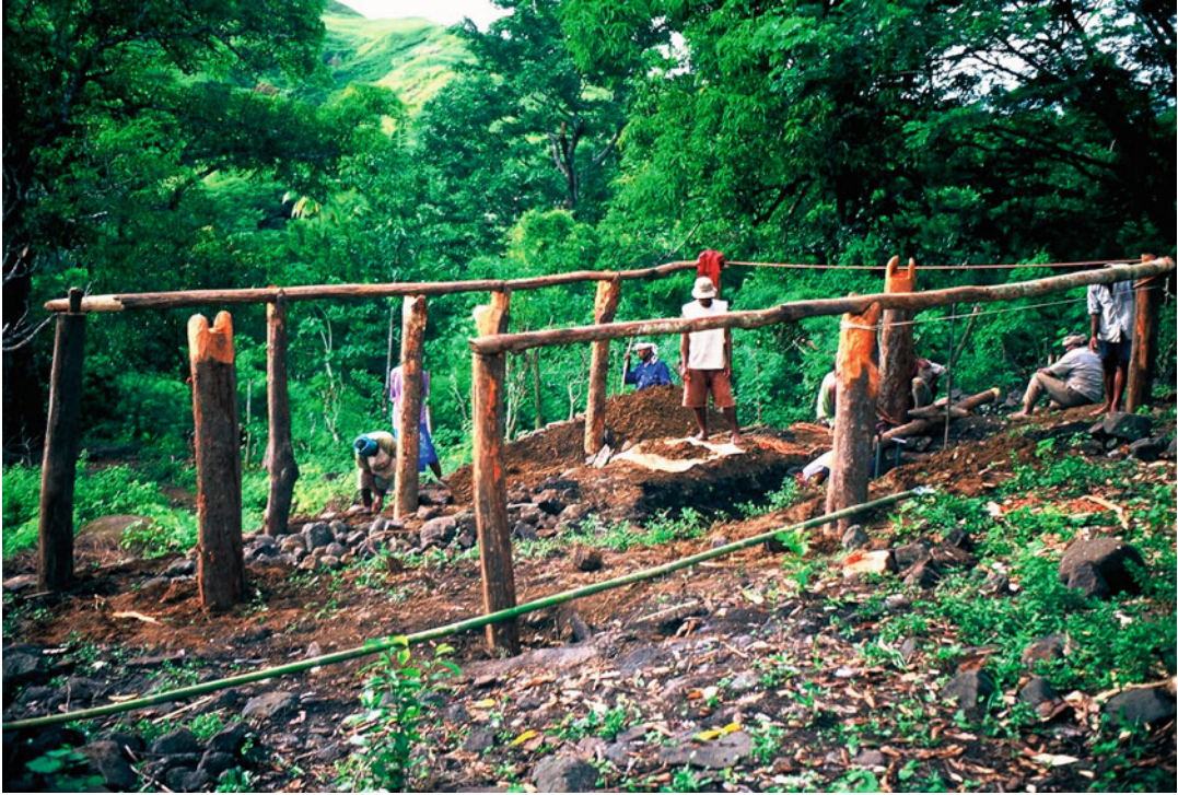
Architecture of Fiji, Fig. 31 Piles dug into the ground before the house platform (Yavu) is erected
