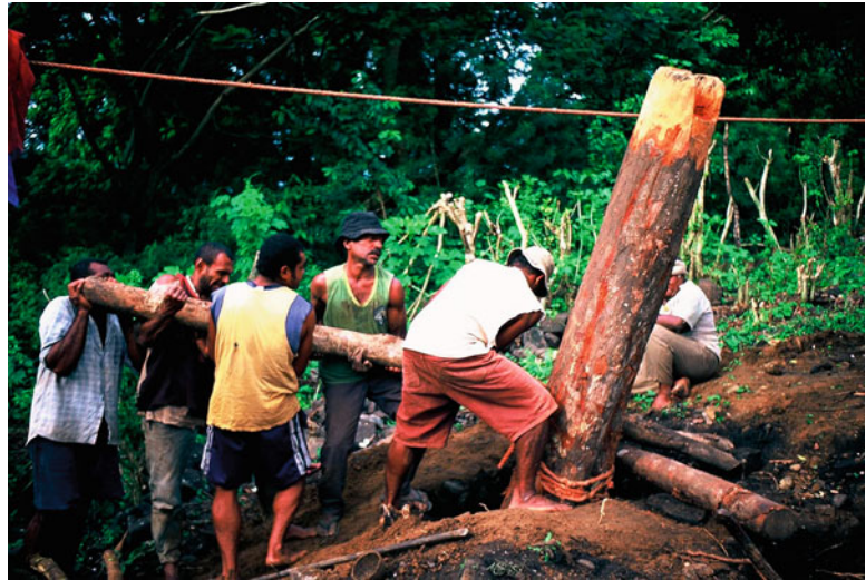
Architecture of Fiji, Fig. 33 Men in Navala village, Ba lever a large pile of a house under construction into its final place
