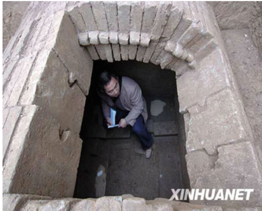
Ancient Urban Water System Construction of China, Fig. 3 Part of the sewer of Han
