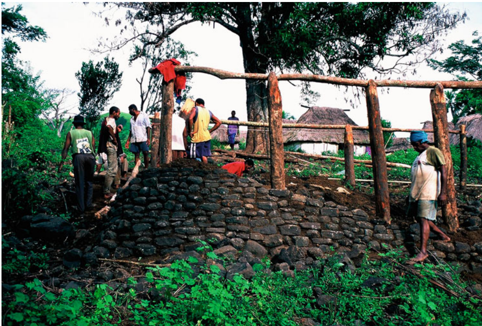
Architecture of Fiji, Fig. 34 The yavu (house platform) is built up after placing the piles
