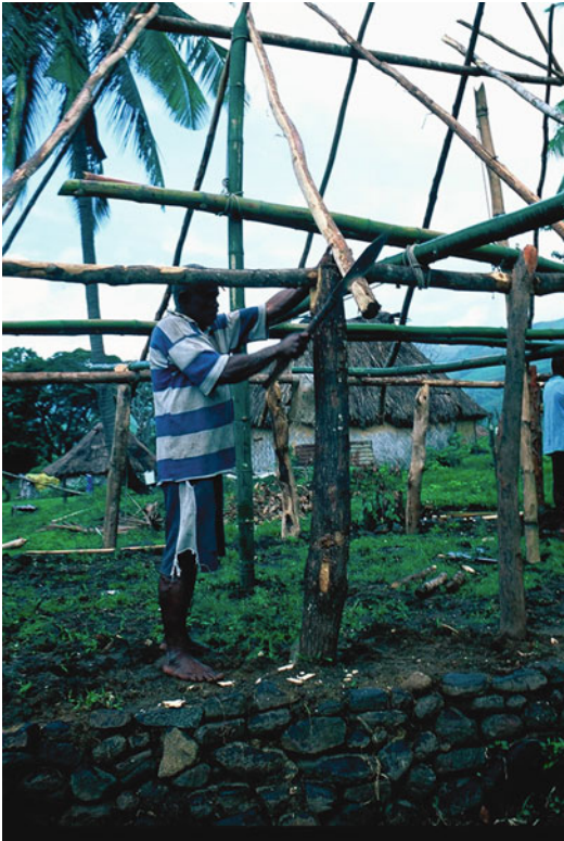
Architecture of Fiji, Fig. 37 The length of the rafters is not calculated exactly beforehand, but they are trimmed after they have been placed in the structure
