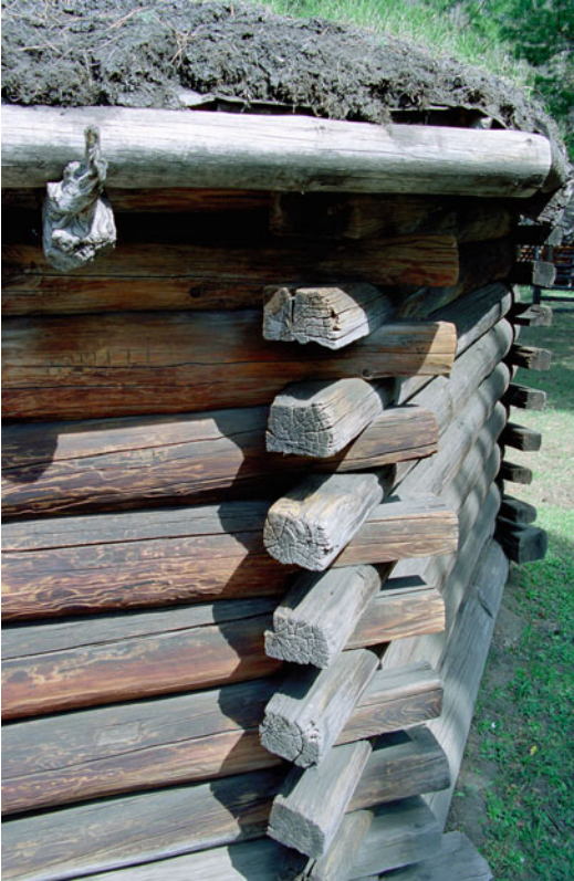
Architecture: Nomadic Architecture of Inner Asia, Fig. 46 Corner detail of a Buriat log cabin
